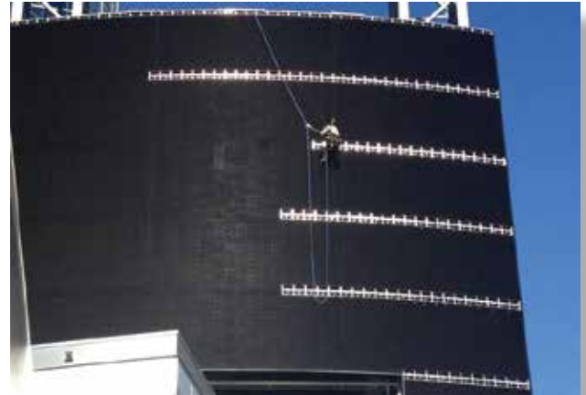
A worker installs panels on a large-scale sign in desert heat; this is a job for Weld-On 30! With its superior sag resistance, big vertical areas are no problem; nor is the desert heat.
